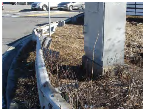
Image 12: Guardrail Damage on the Southwest Corner of the Intersection with Beaver Street and Fortune Boulevard
